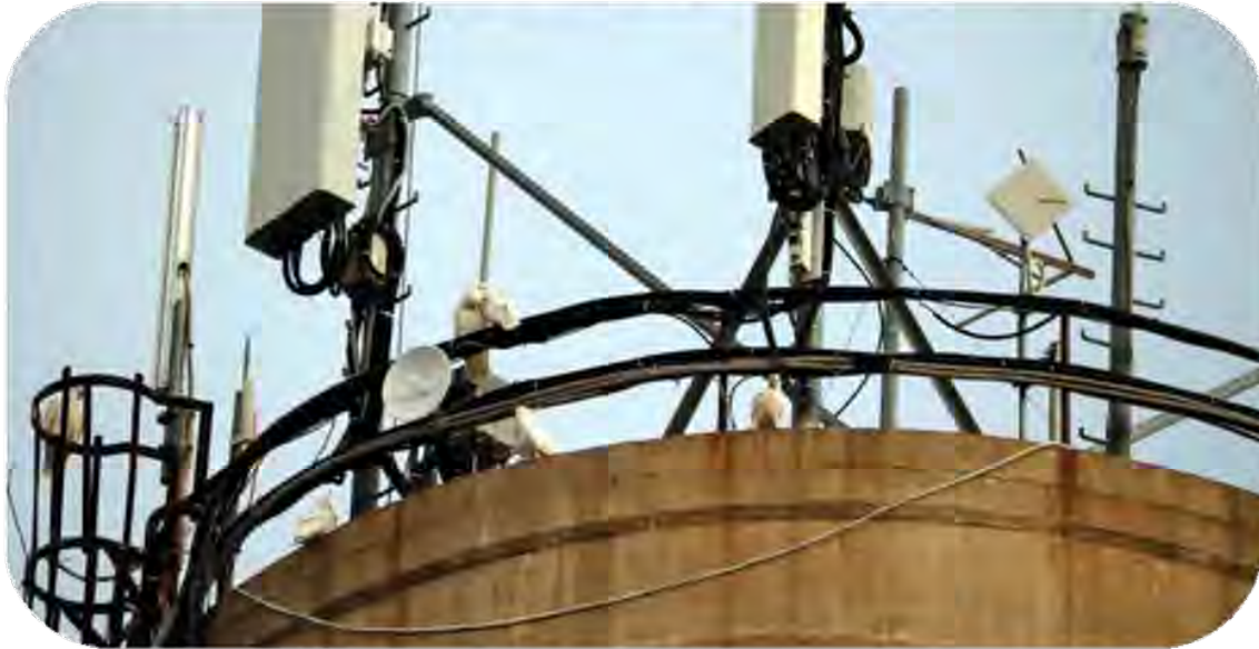
Balonne Shire mobile towers. Credit: SWQROC.
