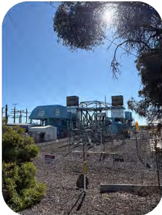
Roma power station, the site of Australia's first commercial gas project. Credit: The Next Economy.
