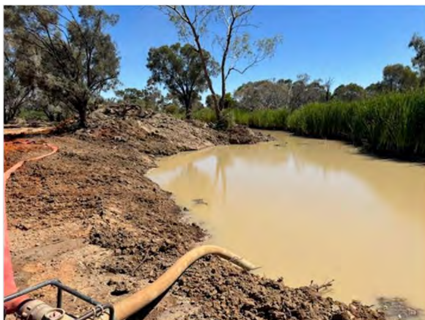
Photo above shows water source opened up to allow for further major construction works in the area.
