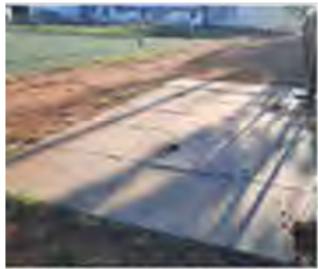
12 PAVED HARDSTAND AT BASKETBALL/NETBALL COURT SERVES NO PURPOSE AND HAS BEEN DAMAGED BY RECENT FENCE CONSTRUCTION WORKS – TO BE REMOVED
