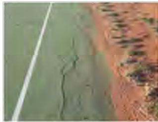
12 BASKETBALL/NETBALL COURT PAVING REACHES END OF LIFE (CRACKED CONCRETE AND GRASS EMERGING IN CRACKS AND UNSAFE TO PLAY ON) – REPLACE OR REPURPOSE SPACE
