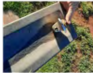
23 DRINKING FOUNTAIN DOES NOT FUNCTION ADEQUATELY – REPAIR OR REPLACE
