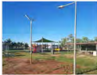
22 LIGHTING IN PARK APPEARS NOT LOGICAL - RATIONALISE
