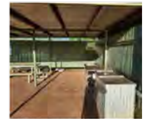
20 LARGE PICNIC SHELTER IS CLOSED IN ON TWO SIDES AND PREVENTS VENTILATION AND BECOMES HOT – REPLACE
