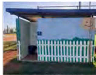
18 OLD AMENITY BLOCK DOES NOT SERVE PURPOSE WITH NEW ONE INSTALLED – REMOVE
