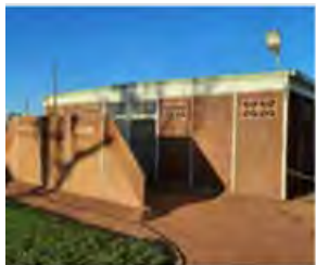
6 CHANGE ROOMS AND AMENITIES FOR PLAYING FIELD HAVE REACHED END OF LIFE AND LOOK OUTDATED - RENEW
