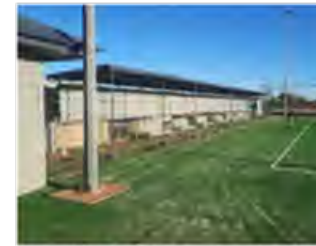
14 TENNIS COURT SPECTATOR SEATING OUTDATED – NEW CENTRAL SHADE STRUCTURE TO FACILITATE BOTH TENNIS COURT AND PROPOSED MULTI COURT
