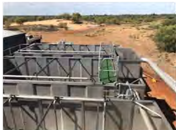
Middle and bottom: Paroo Shire's sewage treatment plant in Cunnamulla, a rotating biological contactor, as proposed for Quilpie.
