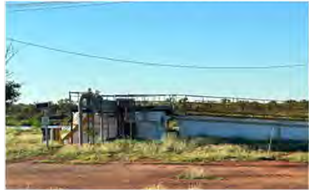
Above: Quilpie Shire's current sewage treatment plant.
