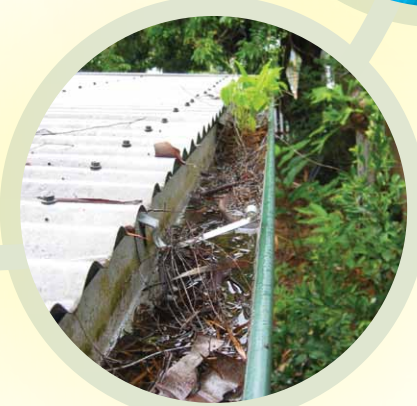
Gutters Clean regularly
